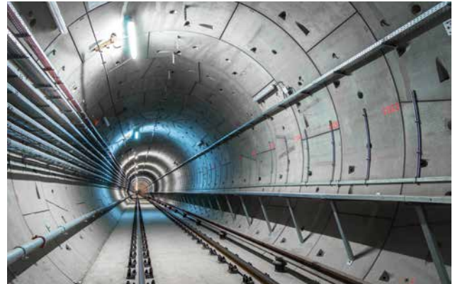
FIGURE 2: EXAMPLE OF FIT-OUT SERVICES.
