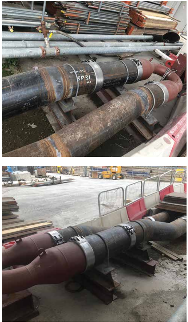
FIGURE 15: EXAMPLE OF 350NB MECHANICAL BODY GRIP RING COUPLINGS ON SLURRY PUMPING LINES
