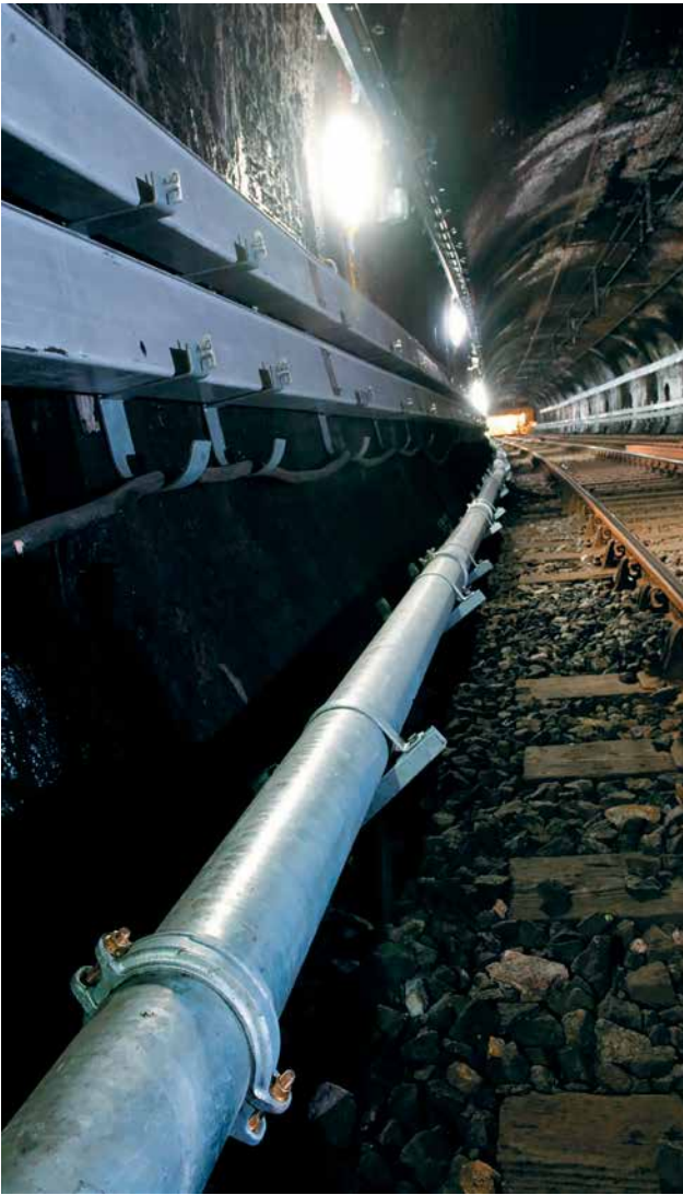
FIGURE 14: EXAMPLE OF GROOVED COUPLINGS BEING USED ON 150NB FIT-OUT WATER SERVICES
